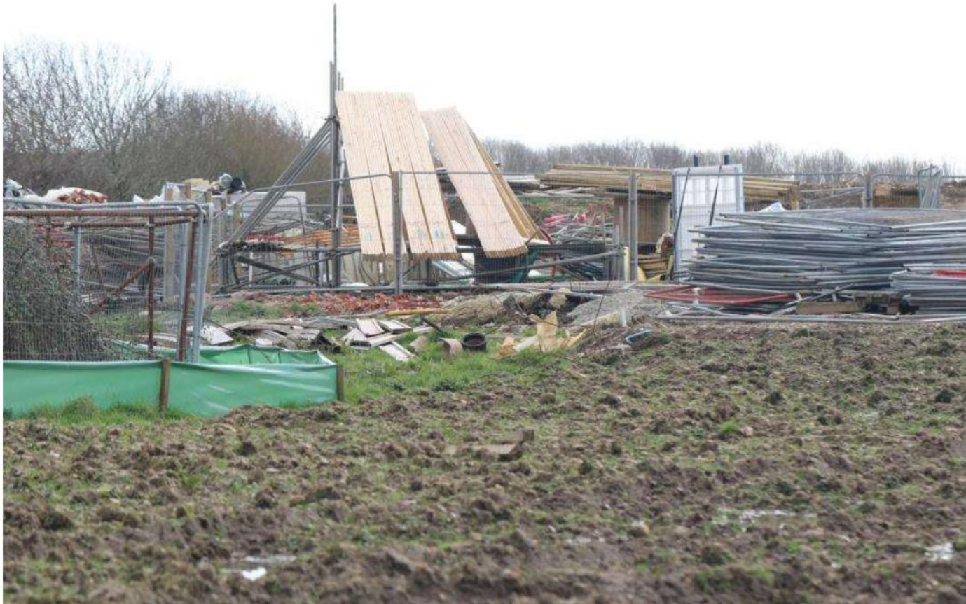
Figs. 9 & 10. March 2020 Immediately above and next page, work continued in fits and starts, with the field to the east here (Map area 6) being accessed for stored materials.
